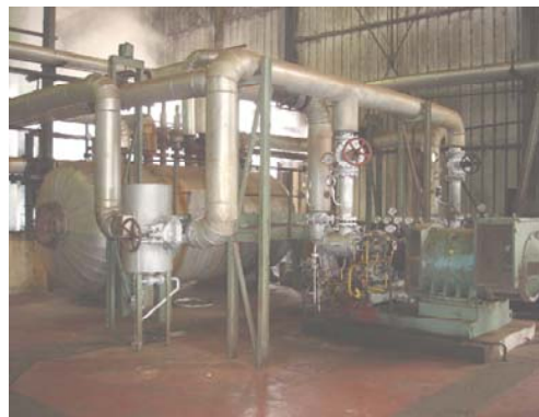
Power generation in a palm oil mill
